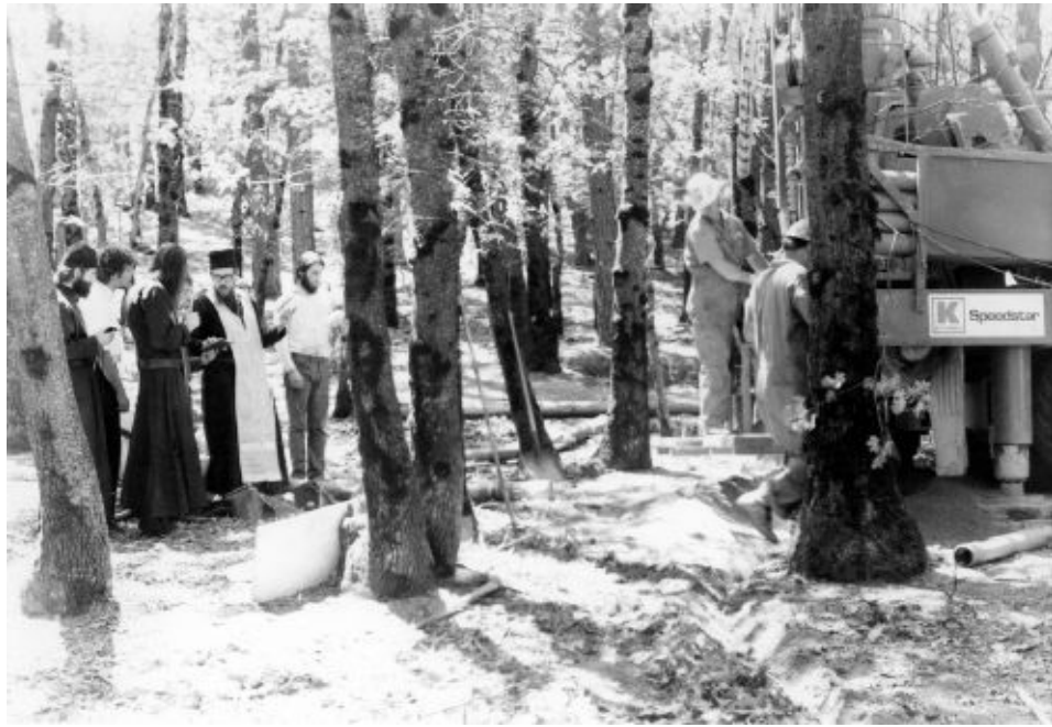
The drilling of the monastery well, while the fathers hold a service of prayerful supplication, July 13, 1977.
